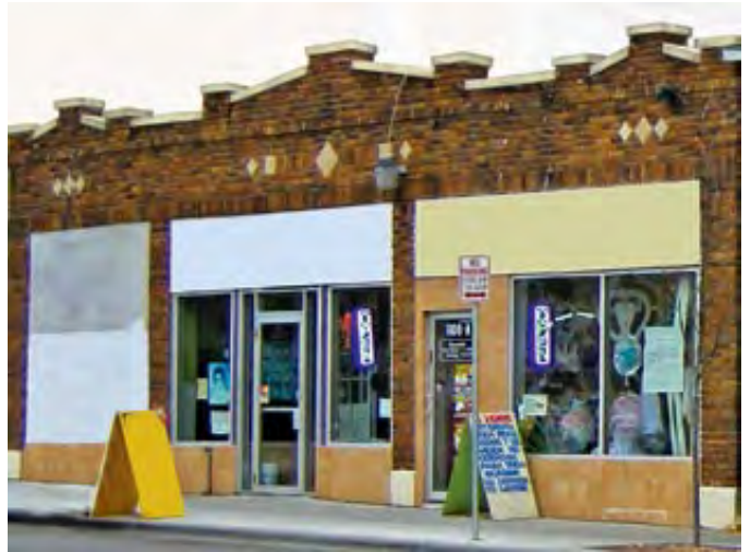
Illustration: Historic building where a storefront window, sign panels and skirtboard panels have been modified in a manner that is not consistent with the building's historical design.
