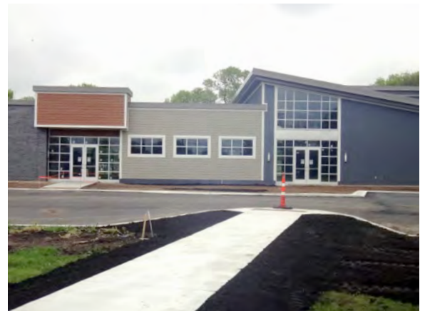
The new City of Rogers Event Center as it neared completion in June 2020.
