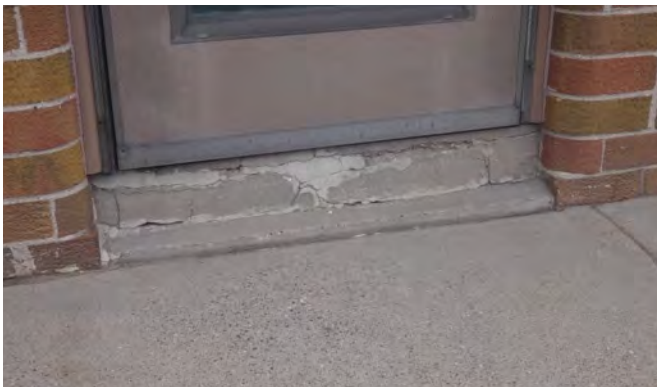
Entryway detail for a historic building along Main Street posing a barrier for wheelchair access.
