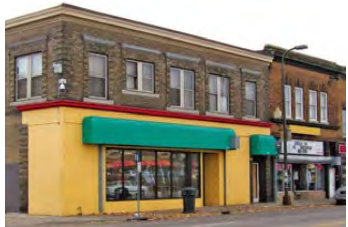
Illustration: Historic building where the original brick wall has been covered with wood siding and then painted, and a non-compatible canopy has been added.
