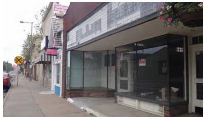
Main Street building with fairly intact major façade elements but with need for rehabilitation of details.
